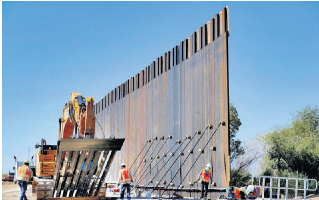
In this Sept. 10, 2019 file photo, government contractors erect a section of Pentagon-funded border wall along the Colorado River in Yuma, Ariz.
